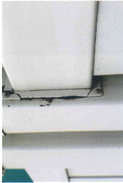
Broken front gate
